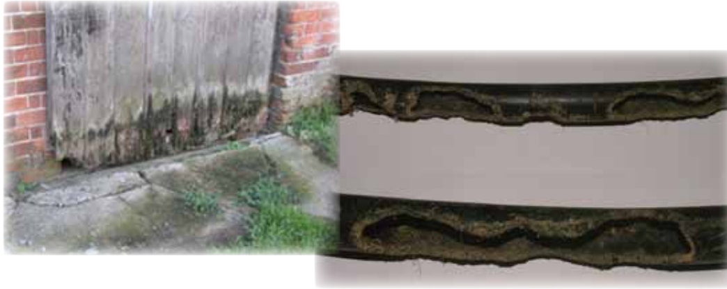
Entry holes and broken pipes are key to fix
